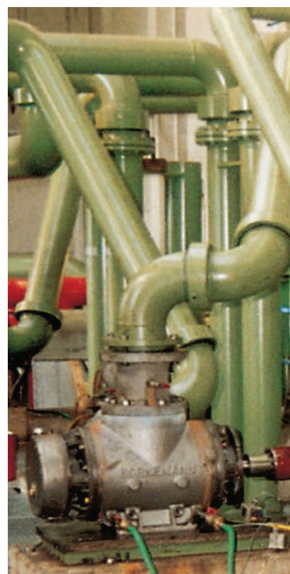
STENFLEX® Swivel Joint type DG-01 installed in a pump test facility
