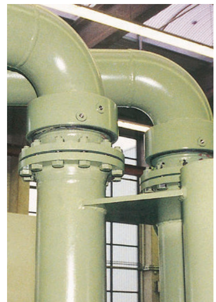
STENFLEX® Swivel Joints type DG-02S installed at loading arms
